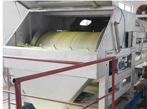
Chemical granulation system
